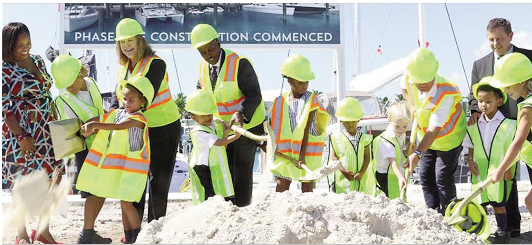
▶ Students of St. Andrew's School help to turn the soil as ground is broken for Palm Cay's One Marina. Also shown from left are Tameka Cartwright, Director of Development and Public Relations, St. Andrew's School; Diane Holowesko Dunkley, chairman, Town Planning Committee; the Hon. Desmond Bannister, Minister of Public Works; Rob Batchelor, Palm Cay and Andy Wood, Principal, St. Andrew's School. (BIS photos/Raymon Bethel Sr.)
