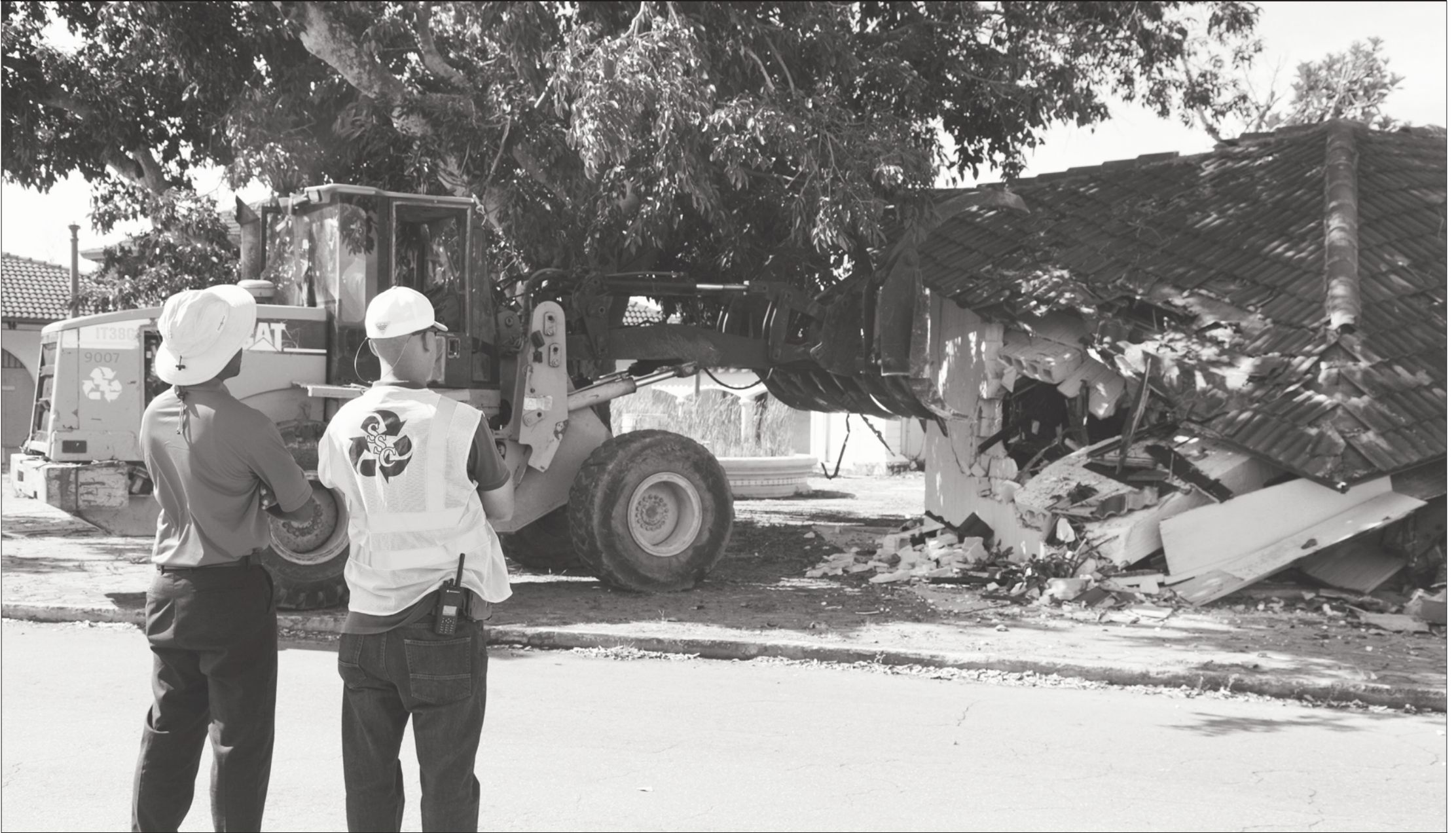
► August 30th, 2018, GBPA and Sanitation Services began the demolition of the burnt straw market located at The International Bazaar. The site, destroyed by fire earlier this year, had become an unauthorized dumpsite and eyesore in Grand Bahama. Pictured L-R: Rico Cargill, Senior Environmental Inspector, Building and Developments Services Department, GBPA; Jason Albury, Landfill Manager and Landscaping and Heavy Equipment Coordinator, Sanitation Services Company.
